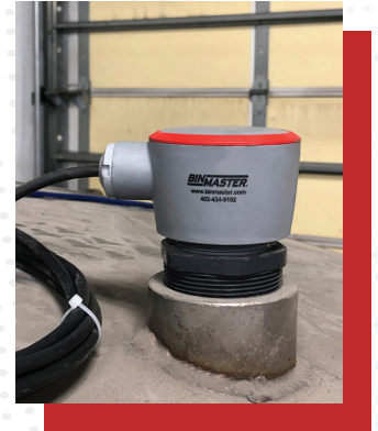
CNCR-130 installed on a fertilizer bin
