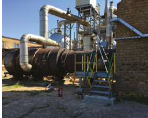
One of the four tail gas incinerators converting remaining sulfuric compounds to SO 2 . The brick structure to the right is the base of the stack, another incinerator feeding the same stack is located further to the right (outside picture). The picture was taken during the installation, hence the ladder on the platform and the fire extinguishers (mandatory, ATEX-classed environment!) on the ground. An RE060 can be seen behind the ladder.
