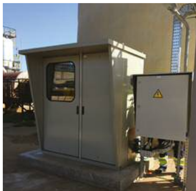
One of the two instrument shelters. The shelter is fed by clean air and kept at a slight over-pressure in order to protect equipment from direct contact with the corrosive atmosphere. Pressure monitors trigger alarms in case of lost over-pressure.
