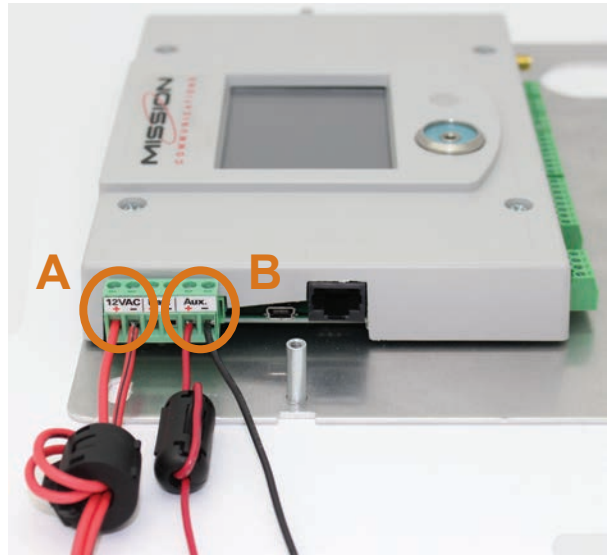
Figure 4: Installing ferrite cores to (A) AC output and (B) auxiliary input
