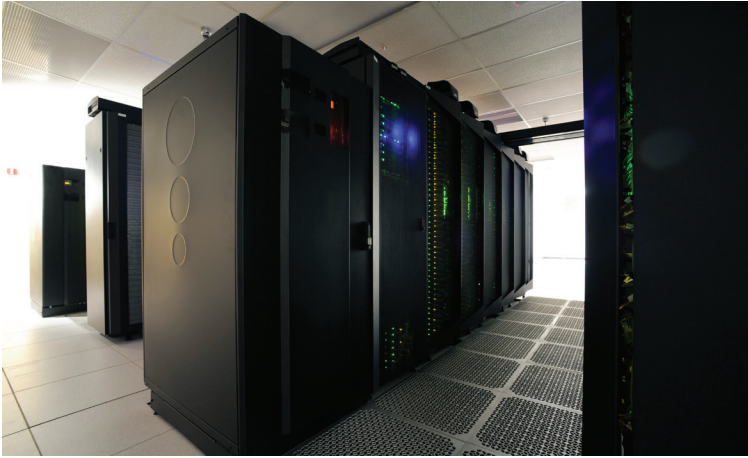
Mission operates its SCADA service from a carrier grade data center located near Atlanta, Georgia.
